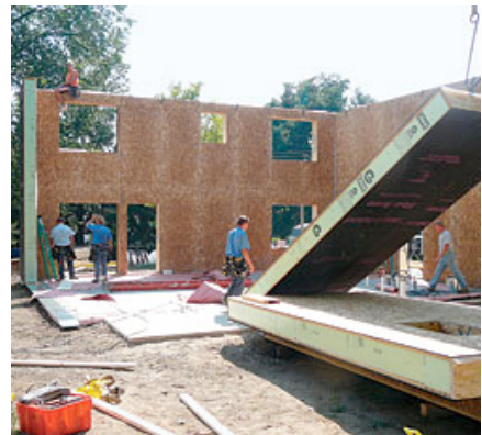
Superinsulated walls are as thick as floors. Built in a warehouse, the R-60 walls are framed with I-joists, insulated with blown-in fiberglass, and skinned on both sides with oriented strand board. They're then delivered to the job site and hoisted in place with a crane.
